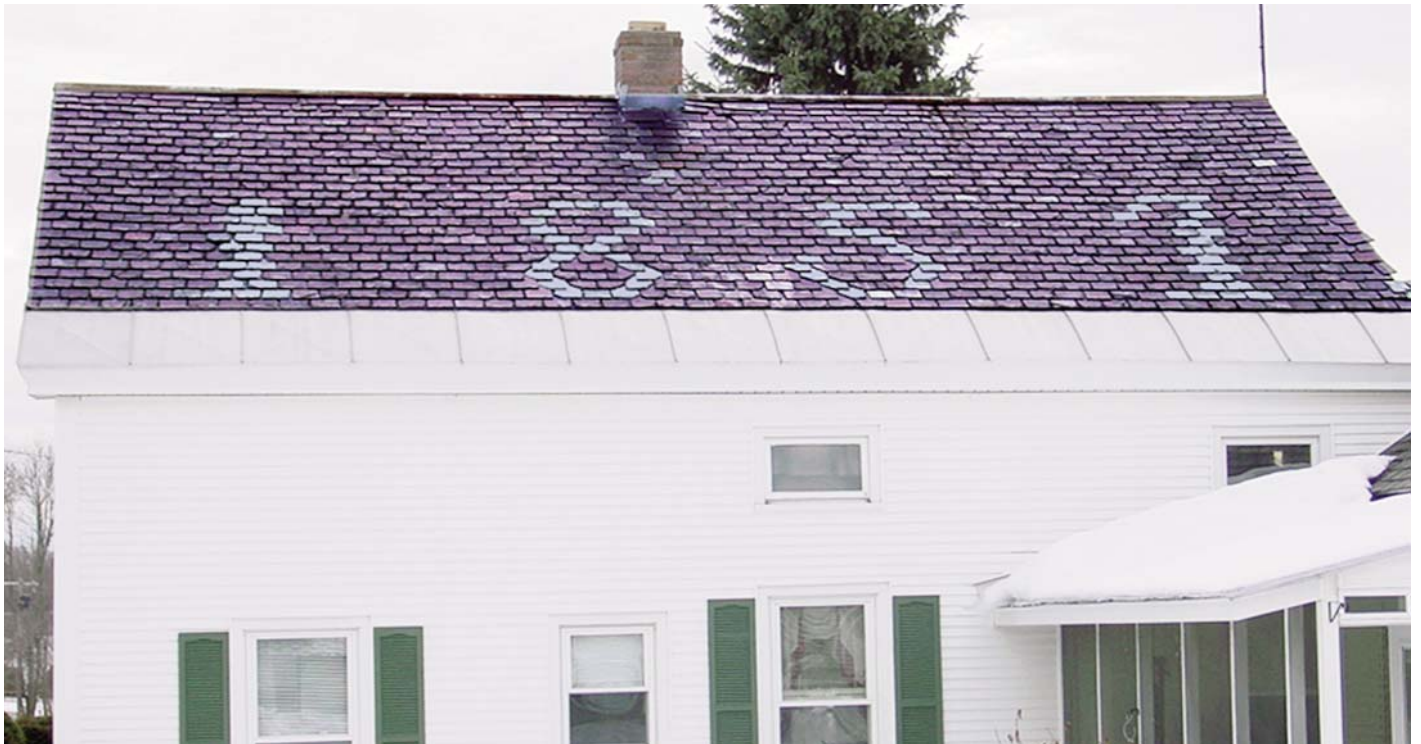
This 150-year-old roof was built of Vermont slate on wood decking and probably nailed with hot-dipped galvanized nails.
